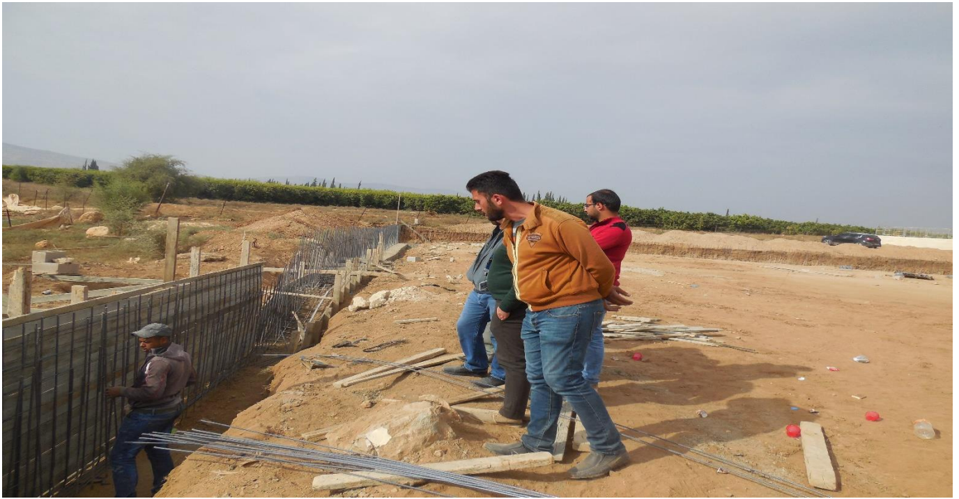
Athletic Field during the first phase of infrastructure – Ein Al Beida, Tubas Cluster
